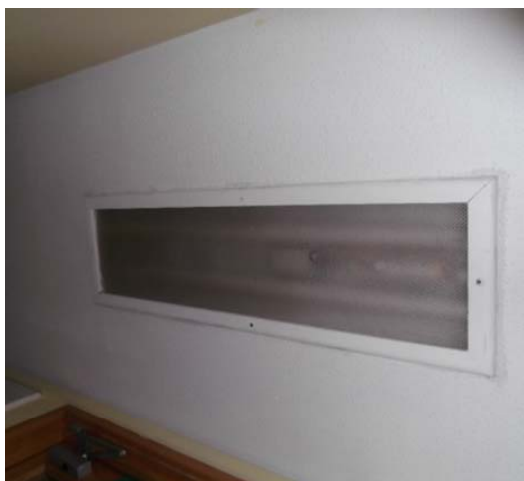
Figure 2: Exemplar undamaged light fitting
